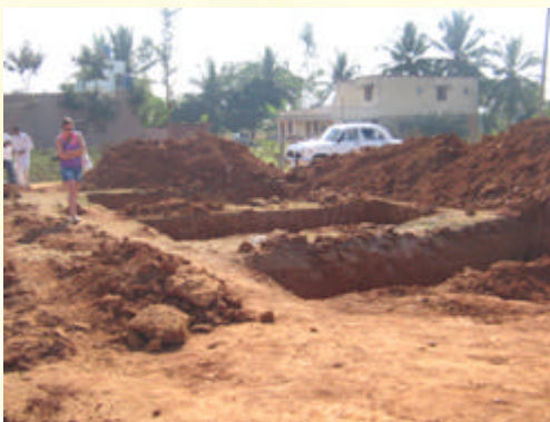
Shreyas Guest, Alexandra Longmore can be seen inspecting the work in progress.
