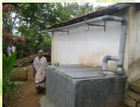
Rain Water Harvesting system at Arjunabittahalli
